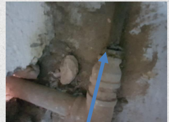
Incorrectly stuffed pipe joint with leak
