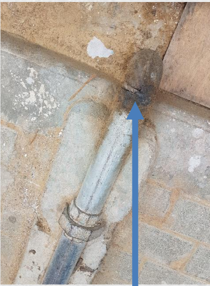
Large mains leak with entirely ineffective attempt at repair
