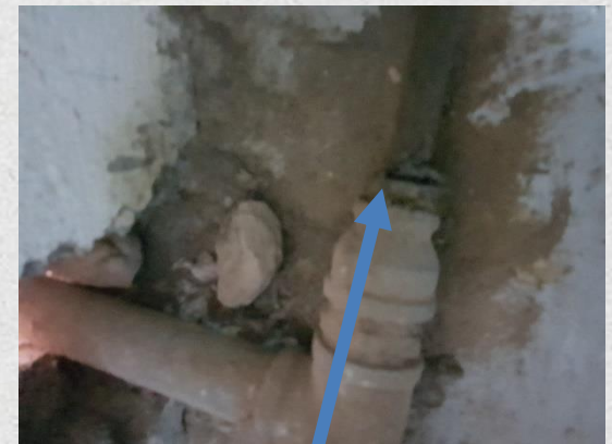
Incorrectly stuffed pipe joint with leak
