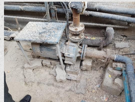
Dirt, clutter and trip hazards.....
